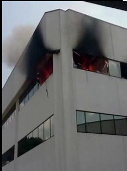
Heavy smoke and flames showing from the fifth floor of the Medical Arts Building in Asheville, NC.
